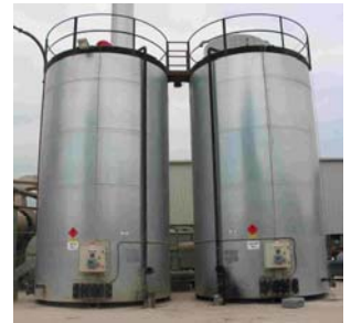
Siemens, Pressvess and BOX ensuring safe handling of HOT bitumen at asphalt sites.
