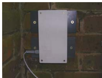
subBOX is that subsidence crack opening or closing?
