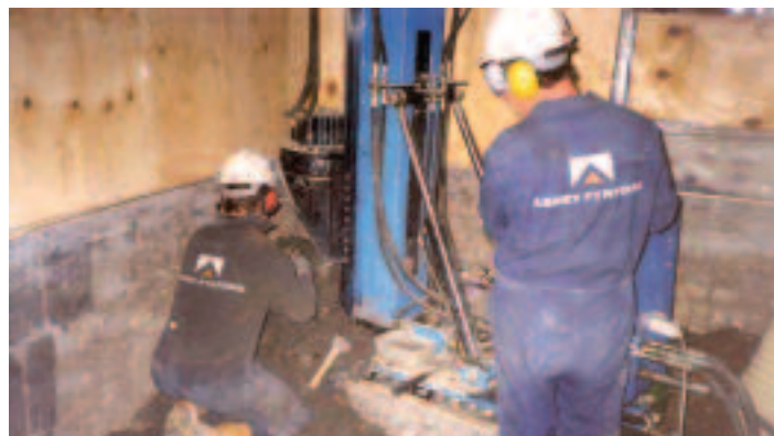
Some piling rigs are small and manoeuvrable for when there is restricted access or low headroom
