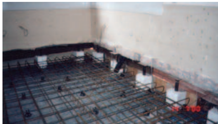
Introduction of a piled raft is one method used to stabilise a property
