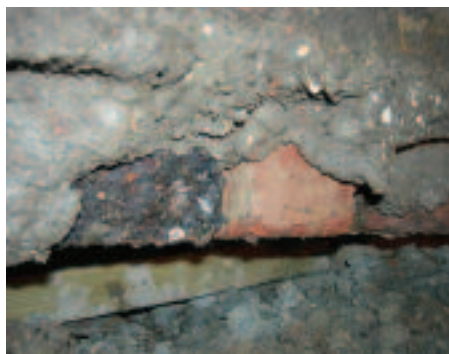
This property was found to be underpinned incorrectly which was the cause of the foundation movement
