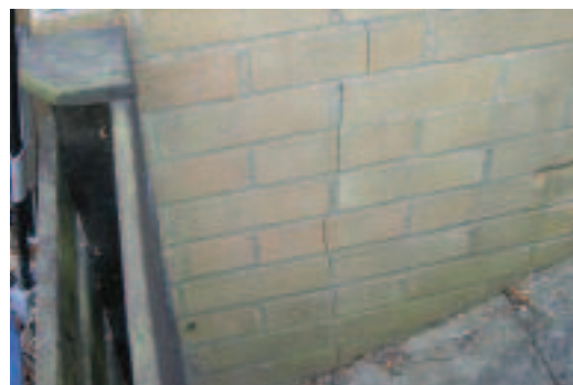
Expansion/contraction cracking – not to be confused with foundation movement
