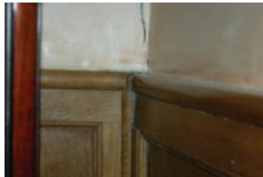
Movement to panelling suggests foundation movement
