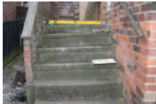
Steps moving due to ongoing compaction of fill material not subsidence – trial holes were critical in proving this
