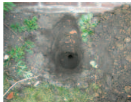
Trial holes at this property revealed the presence of made ground enabling ground movement
