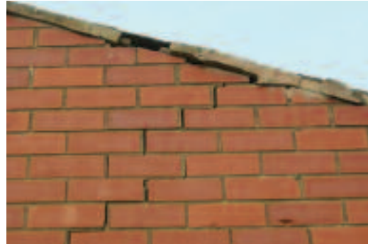
Foundation Movement cracking – diagonal and tapering in width
