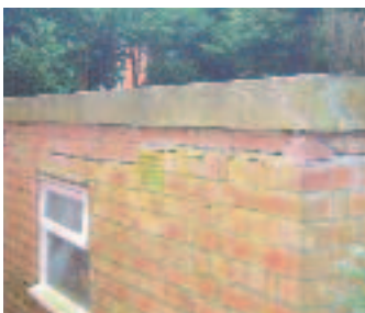
Top to bottom: Damage on rear elevation, pulling around rear elevation window and dragging effect of roof decking (and evidence of previous repairs)
