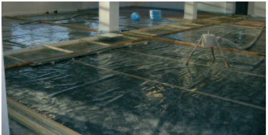
Same office floor about to be repaired using concrete, which should survive any future flooding incident
