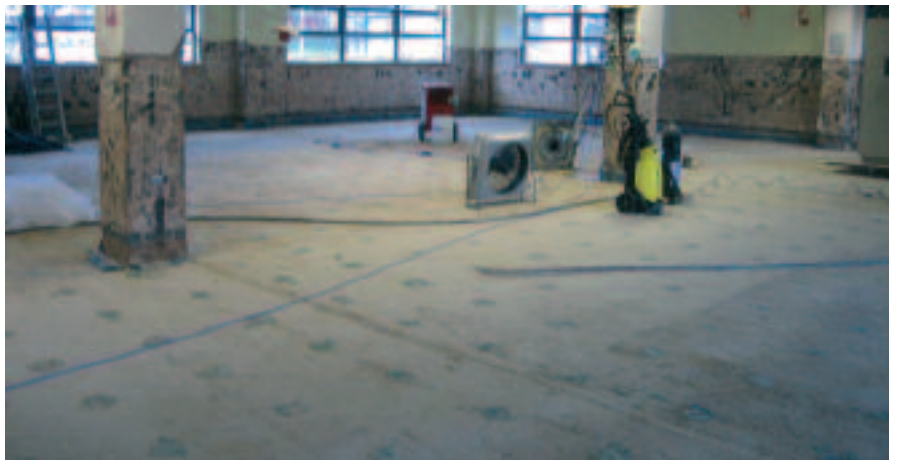
Office floor after flooding with the perished chipboard false floor removed
