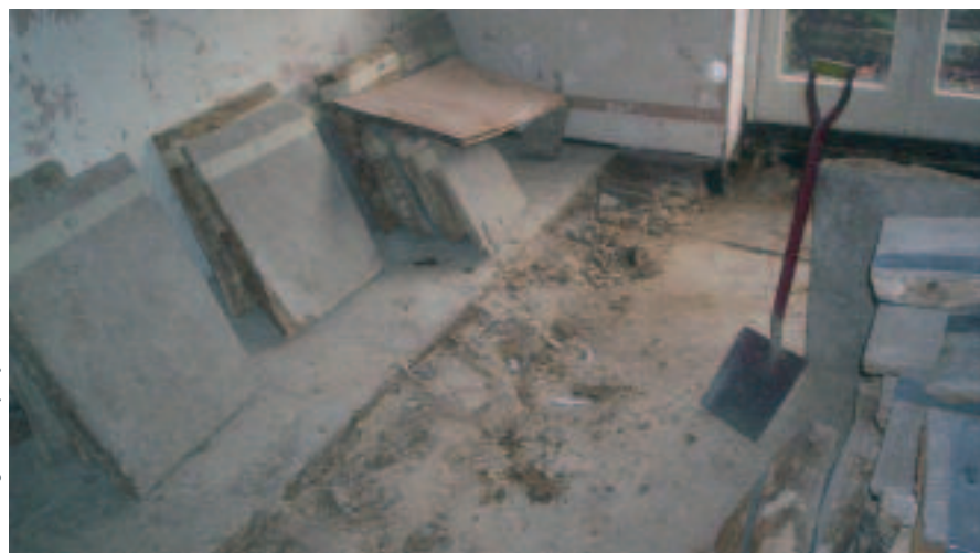
Investigations into a stone flag floor that was not drying out (note the salvaged flags are labelled for precise reinstatement)
